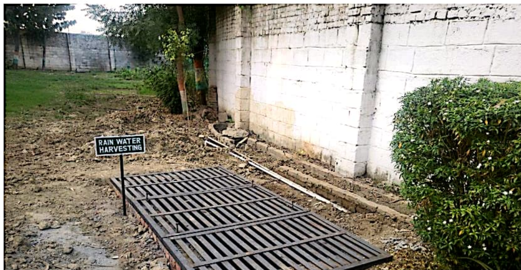
(Rainwater harvesting soaking pits in the campus)
