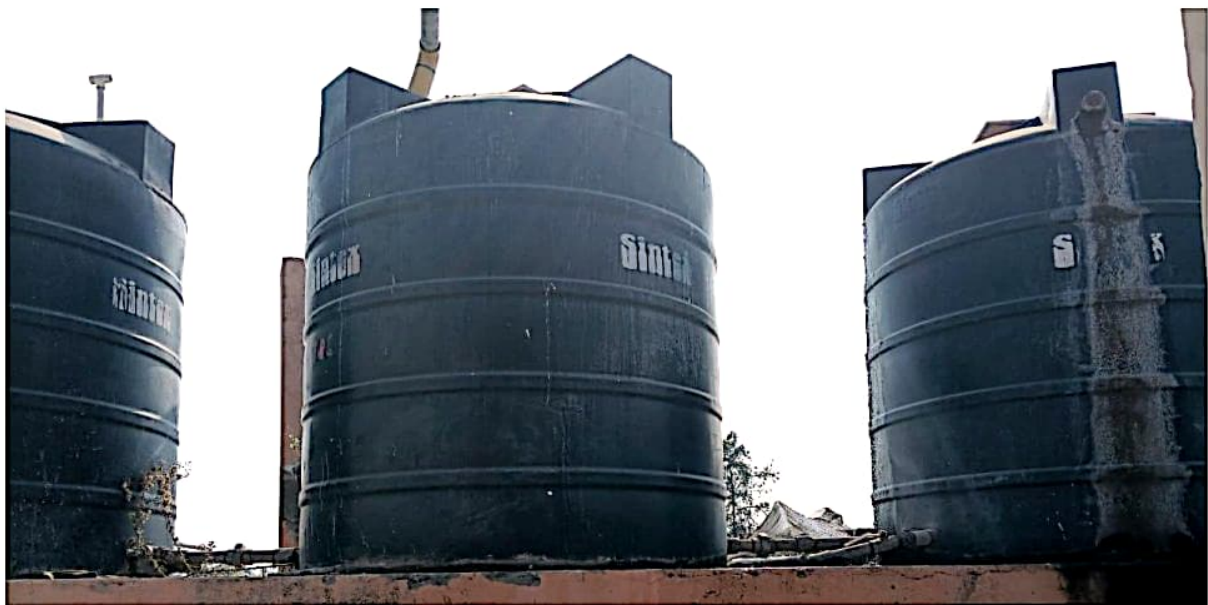
(Multiple overhead water tanks on the rooftop for seamless water supply)
