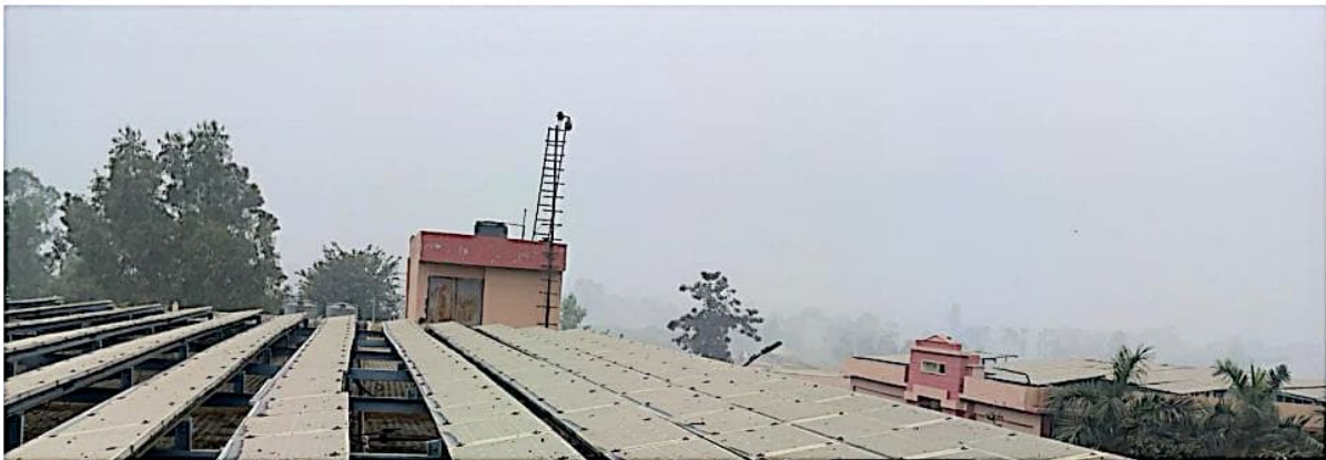
(Solar based energy system in the SUG campus)
