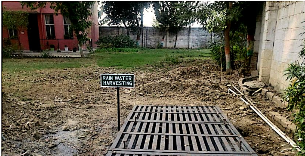
(Rainwater harvesting facility in SUG campus)
