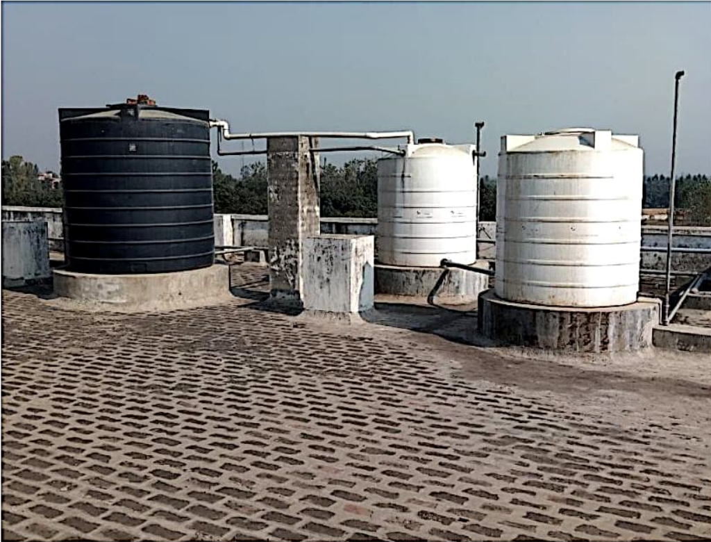
(Multiple overhead water tanks on the rooftop for seamless water supply)
